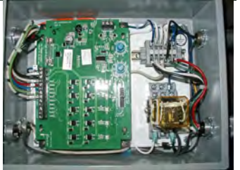
9517 00 Baghouse Timer Box
