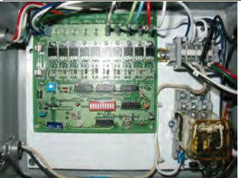
9517 AA Baghouse Timer Box (Old style board)
