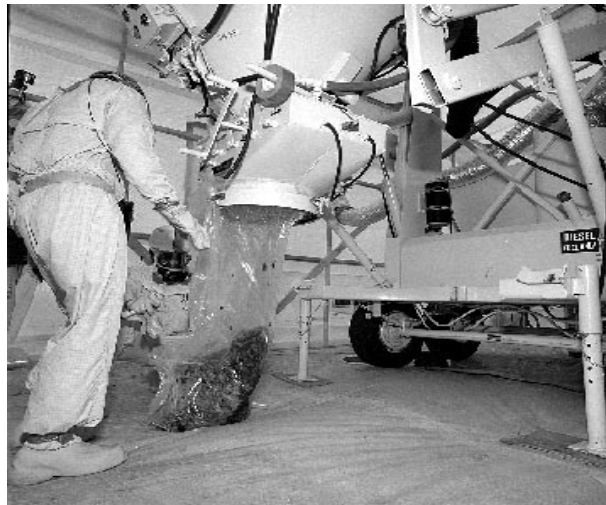
Figure 4. Insulation removed by the VecLoader being discharged by worker into plastic bags.
