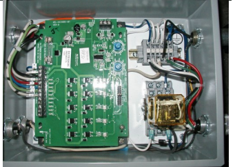
9517 00 Baghouse Timer Box
